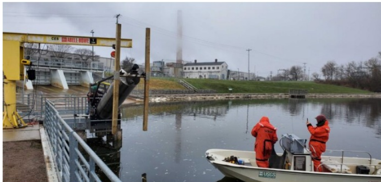
The U.S. Geological Survey watches from a boat as the Archimedes screw is installed. Scott Miehs
